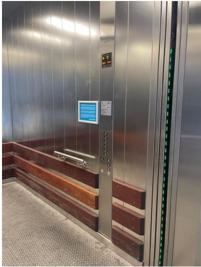
Goods Lift Interior
